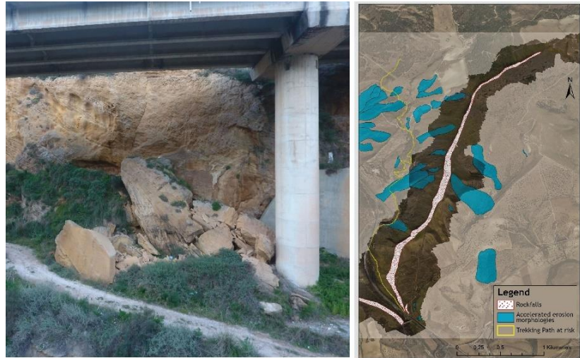
Fig.3: Rockfall January 2007: several blocks rolled down the gorge, stopping very close to the first viaduct pillar and on top of the main natural path (Sentiero Natura). To the right, the elaborated map of visible rockfalls and accelerated erosion affecting the Sentiero Natura. (Photo by Daniele Maglitta)
