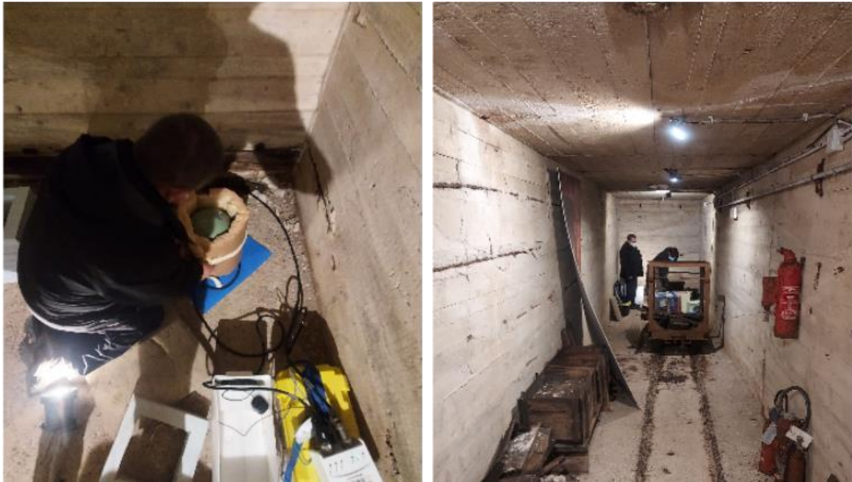
Fig.3: Installation of a broadband seismic station within the Mining Museum (photograph by INGV)
